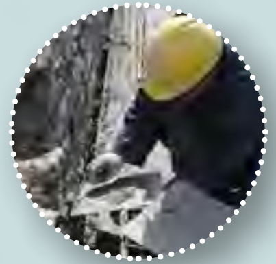
Here, selective pointing is being carried out to facilitate maintenance of access points for bats and birds. Certain gaps can be left without interfering with the structural stability of the building
