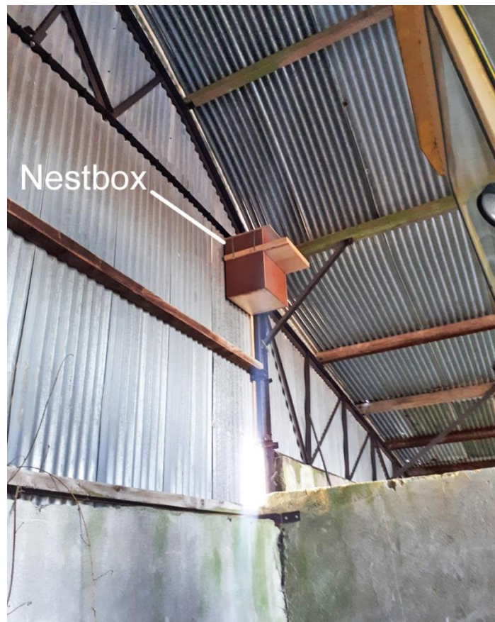
This box is secured using 2 lengths of steel band from one side of the box over the top and into the wooden roof beam (Image: Alan McCarthy)
